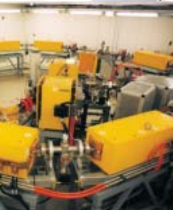
on booster for the ANKA facility
