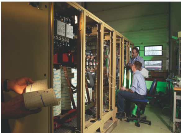
The 3200A / 704 kW dipole magnet power supply
